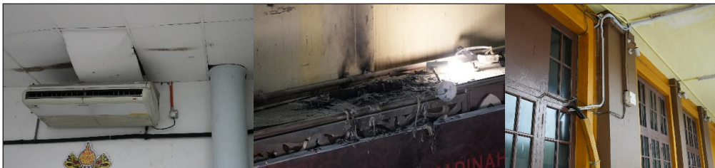
Figure 3. Museum amenities that could potentially cause electrical trips, leading to fires, include unmaintained lighting and outdated wiring systems
